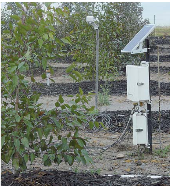
Plate 17. Data Logger for Soil Temperature Probes
